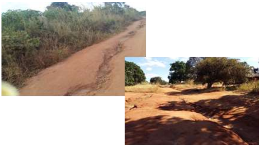
Picture 2-1: Roads condition in Murrumbala and Memba Districts
